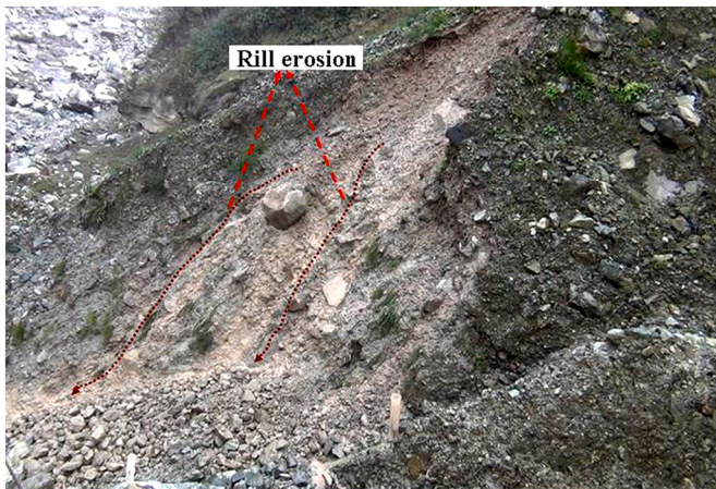
Fig. 5. Evidence of surface flow and rill erosion.
