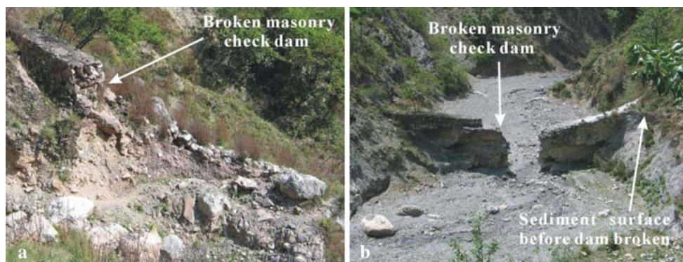
Fig. 5 Site photographs showing two broken check-dams in upstream of Duozhao ravine. a Broken check-dam in Xiaoya channel, position (3,140E–380N), by the impact of dolomite blocks from
