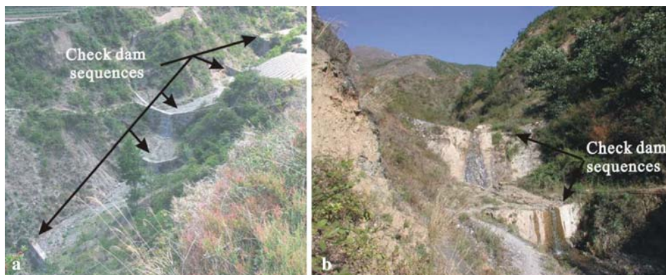
Fig. 4 Site photographs showing sequence of pointed random rubble check-dams in good condition in the debris-flow channels in Duozhao. a Check-dams in Daqishu channel, position (3,240E–2,050N); b check-dams in Dasha channel, position (3,340E–1,310N)
